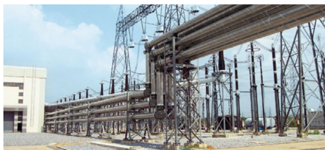
Fig. 2.5-6: Above ground installation
